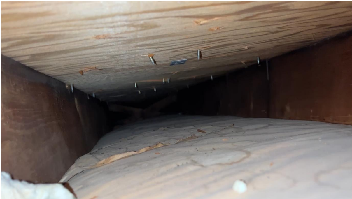
Looking down a rafter bay above the Garage Bedrooms from the Bathroom Attic
