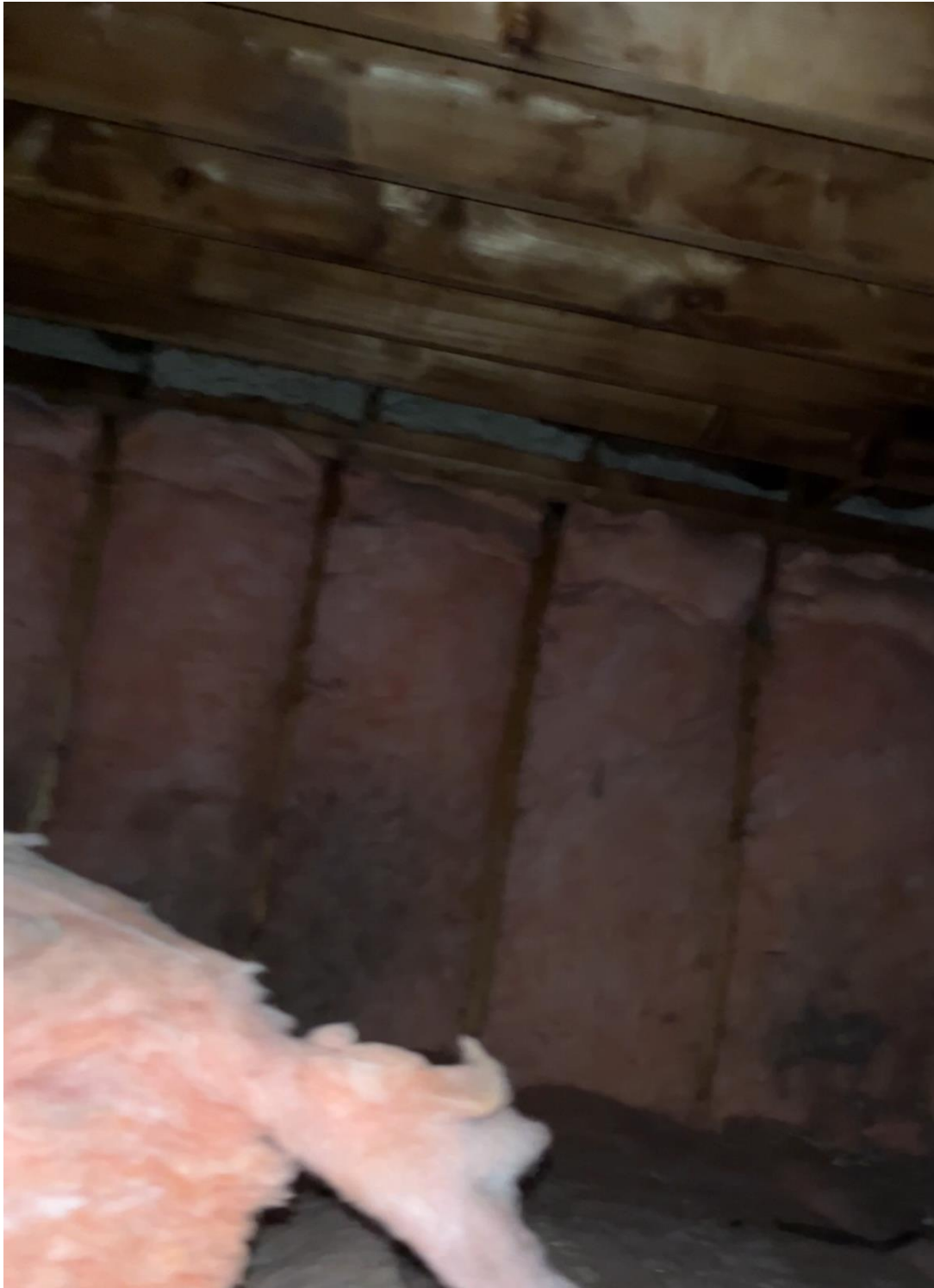
Bedroom Attic space from access hatch in the bedroom ceiling. You can see the White insulation in the rafter bays above the garage bedrooms.
