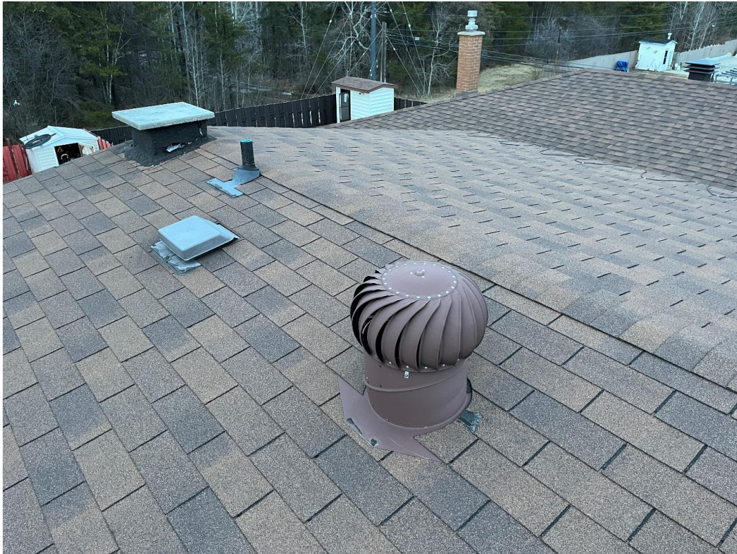
Roof peek, the Garage Bedrooms are on the right. The small vent is above the Bathroom Attic and the turbine vent is above the hallway. Old Chimney will be removed.
