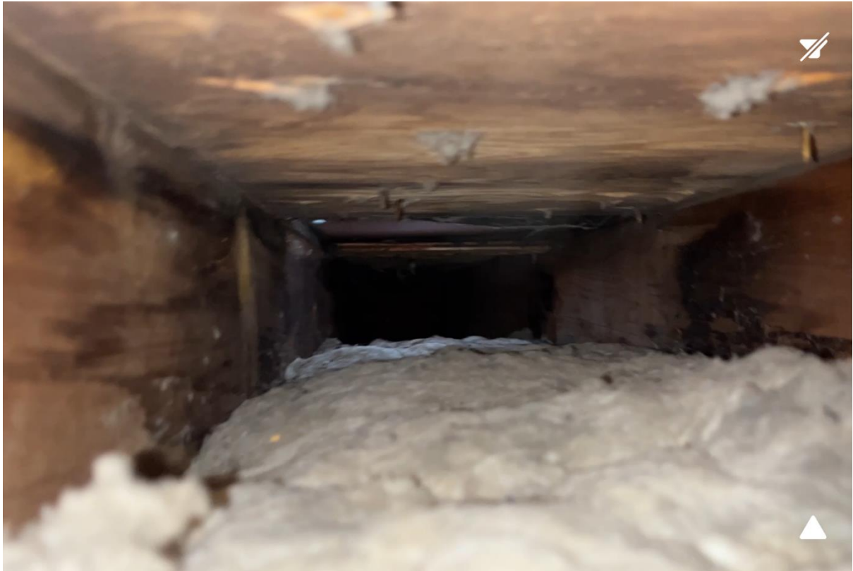
Looking down a rafter bay that crosses from the Bathroom Attic, over the hallway and into the Bedroom attic. You can light from the turbine vent.
