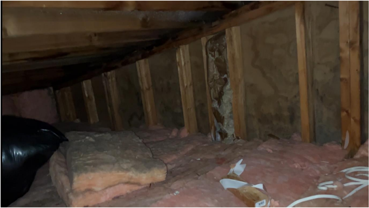
Bathroom Attic Space from the access door that is on the knee wall in a bedroom above the garage. That is the Back Exterior Wall
