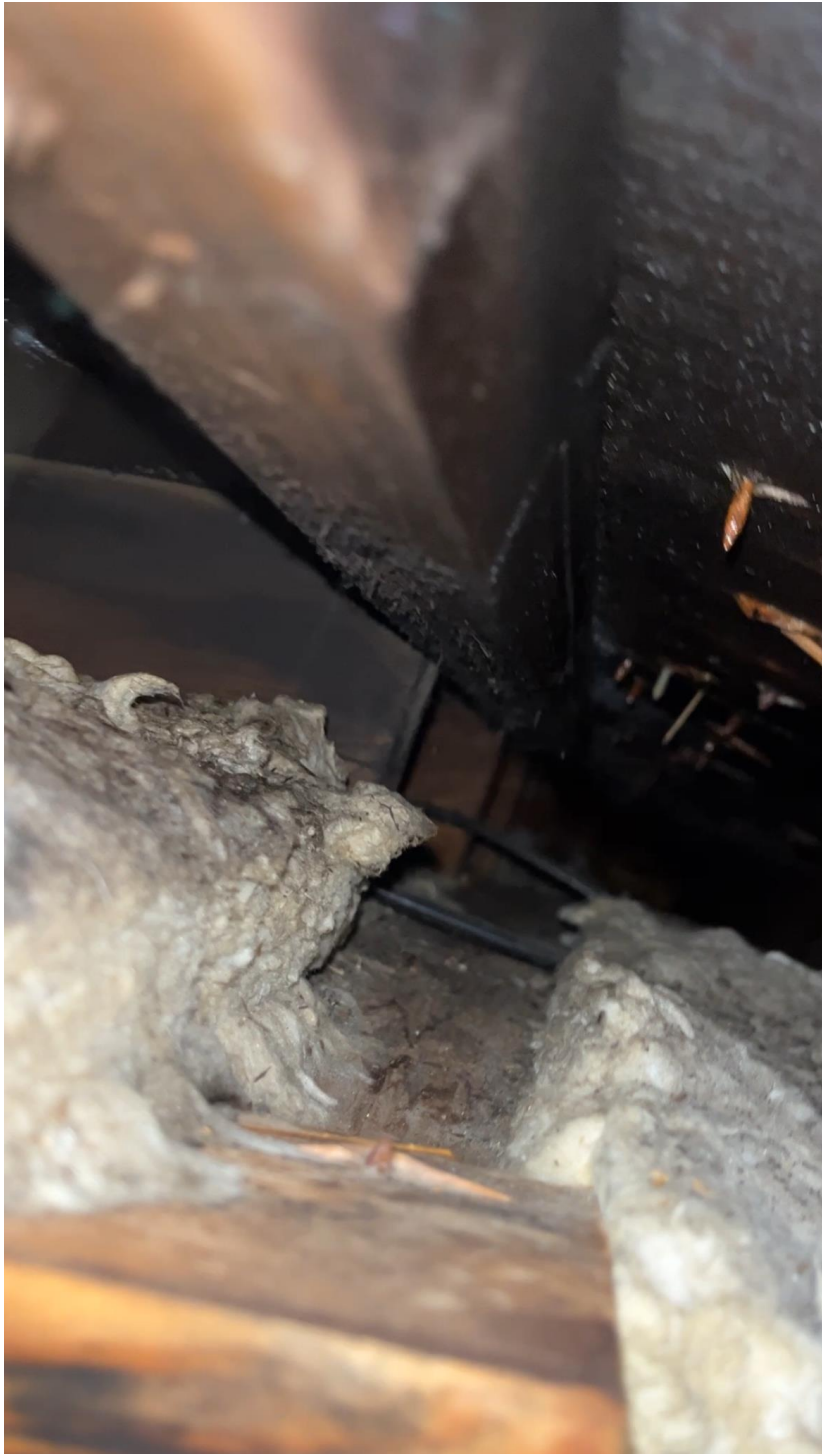
Looking down a rafter bay where all the Garage Bedroom Rafter meet. The view crosses from the Bathroom Attic, over the hallway and into the Bedroom attic.
