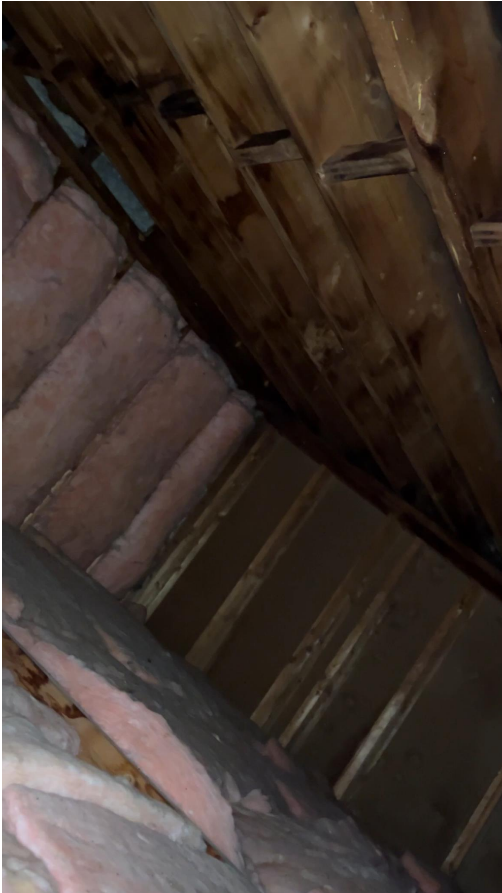
Bedroom Attic space from access hatch in the bedroom ceiling. That is the front exterior wall.
